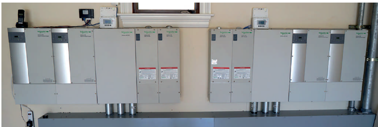
Image: Schneider Electric, a domestic installation for a large house or small commercial application
